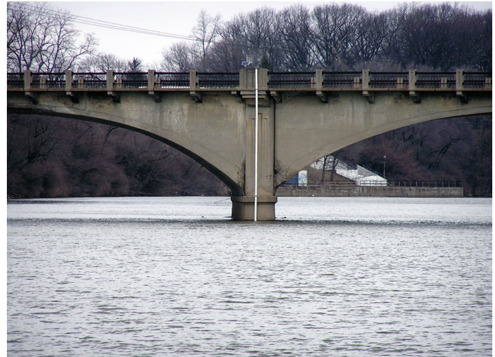
Deployment site for Indianapolis OES. The sonde is deployed in a long PVC tube for protection. The solar panel and telemetry system can be seen at bridge level.
